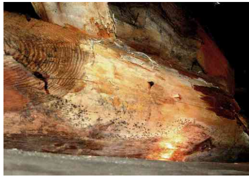
Figure 2 – Soft rot development in poor-ventilated space of wooden structure.
