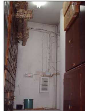
Figure 3- Faulty electrical board in the storage facility
