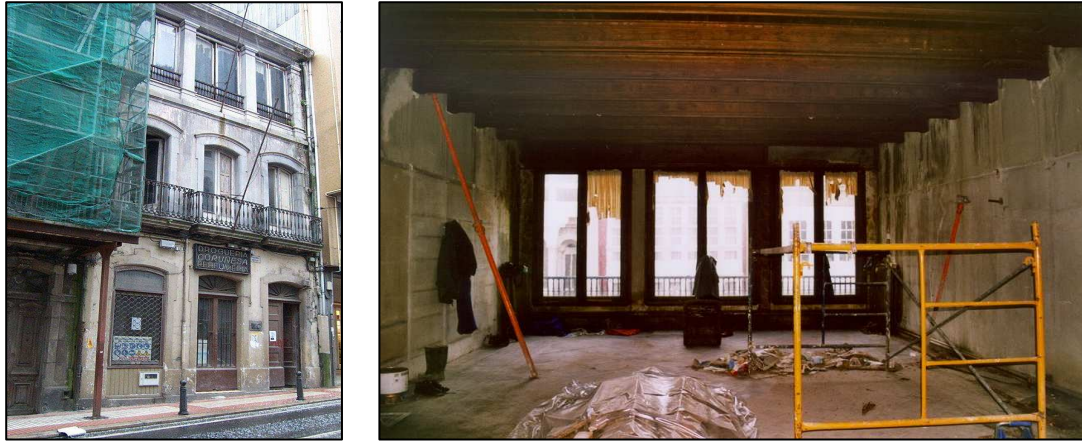
Figure 1. General view of the building and detail of a room where the beams are hidden inside artistic covers.
